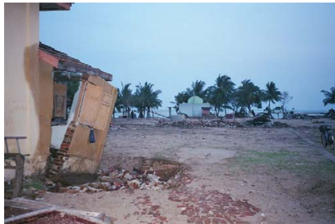
Typical foundation scour resulting in collapse
